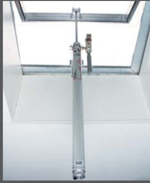
On dome with thermal valve
