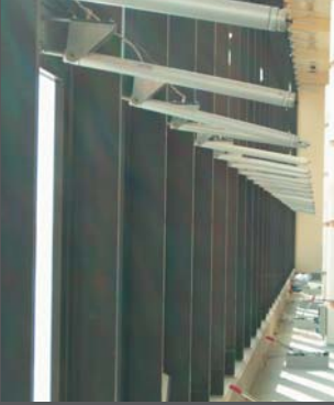
Installation on top hinged window with connection to compressed air system
